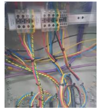
PROFIBUS cable attached to high-voltage
