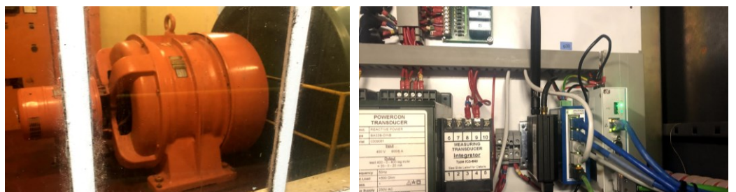
Hydroelectric power generation plant
