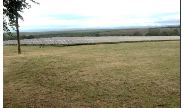
Solar generation farm
